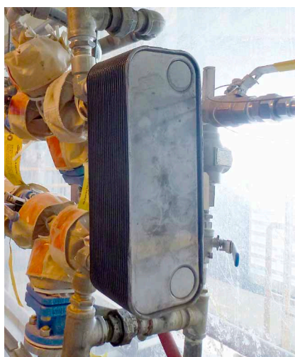
Alfa Laval tantalum heat exchanger installed at PQ Corporation.
