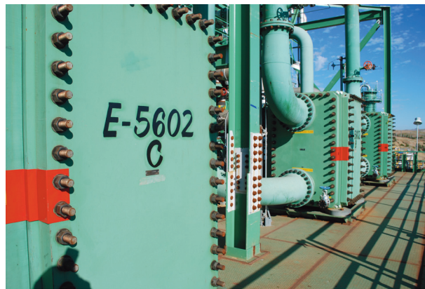
Figure 3. The heat exchangers ensure environmental compliance in a Belco flue gas scrubber (Jim Hill).
