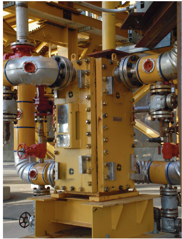
Figure 5. Compabloc heat exchanger recovering heat in a Cansolv lean to rich service (Jim Hill).
