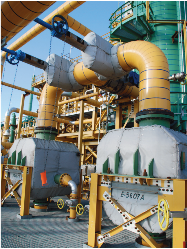
Figure 4. Reboilers efficiently add heat to a Cansolv lean amine stripping tower (Jim Hill).
